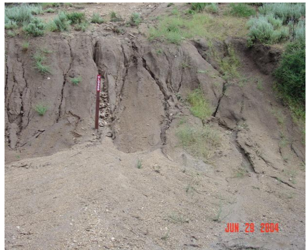
Figure 5. Rill erosion (USDA-Forest Service image).
