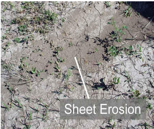
Figure 4. Example of sheet erosion.
