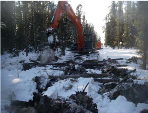
Photo 3: An excavator is used to dig holes and place the soil beside the hole creating an elevated mound. Elevated mounds create an elevated microsite that increases soil temperature and improves growing conditions for natural regeneration and planted seedlings. Mounds can also help create an access barrier for human travel and may impede predator movement on lines.
